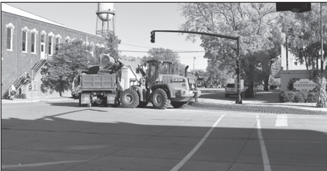
Not the road resurfacing intended While Highway 65 in Northwood will undergo a resurfacing project next year, it will not be made into a gravel road, as it may have briefly appeared recently. A truck carrying gravel left some material behind before the Northwood public works crew was able to get it back into place.
